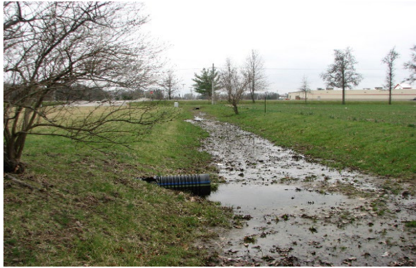
7. View of the drainage swale along the western boundary of the site.
