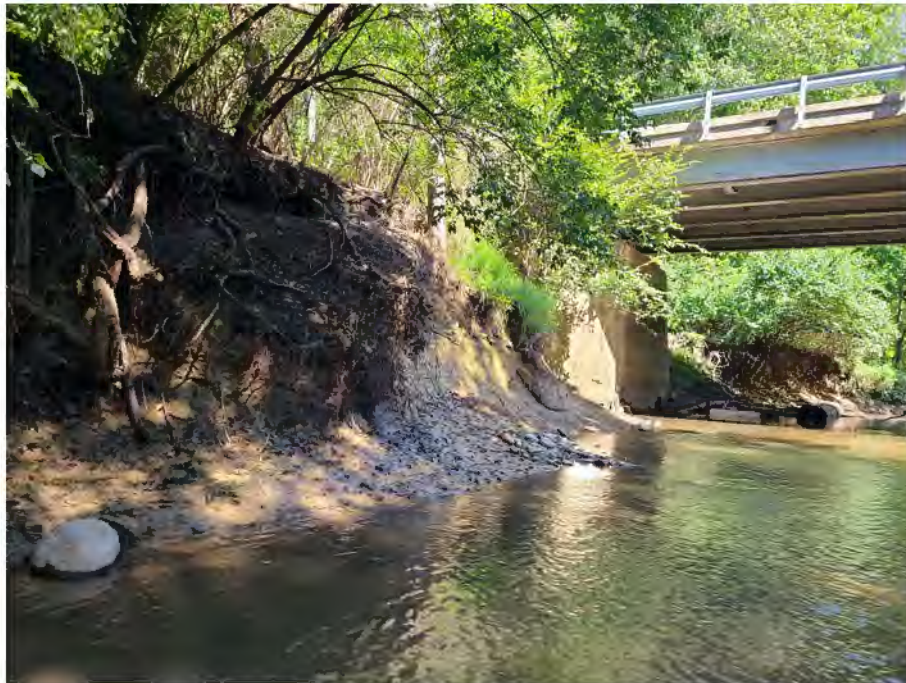
Figure 2. The McLean County Highway 21/2600 E (FAS 489) bridge project, McLean County, Illinois on 8 September 2021. Top image taken from upstream of the bridge, facing north, and shows coarse woody debris accumulation on bridge pylon. Bottom image taken from downstream of the bridge, facing upstream (east), showing scoured banks and hardpan substrate. Photos by A.P. Stodola, INHS.
