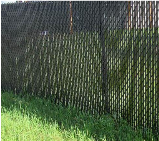
Photo 1. An example of vinyl privacy slats that would be woven into the chain-link fence and would extend to the gravel pad to inhibit turtles from entering the station.
