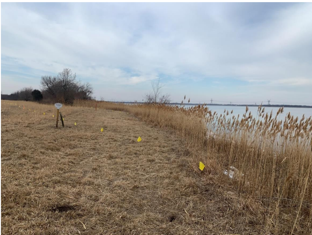
Photo 4. Construction area in the ROW south of Heidecke Lake. Grundy County, IL.
