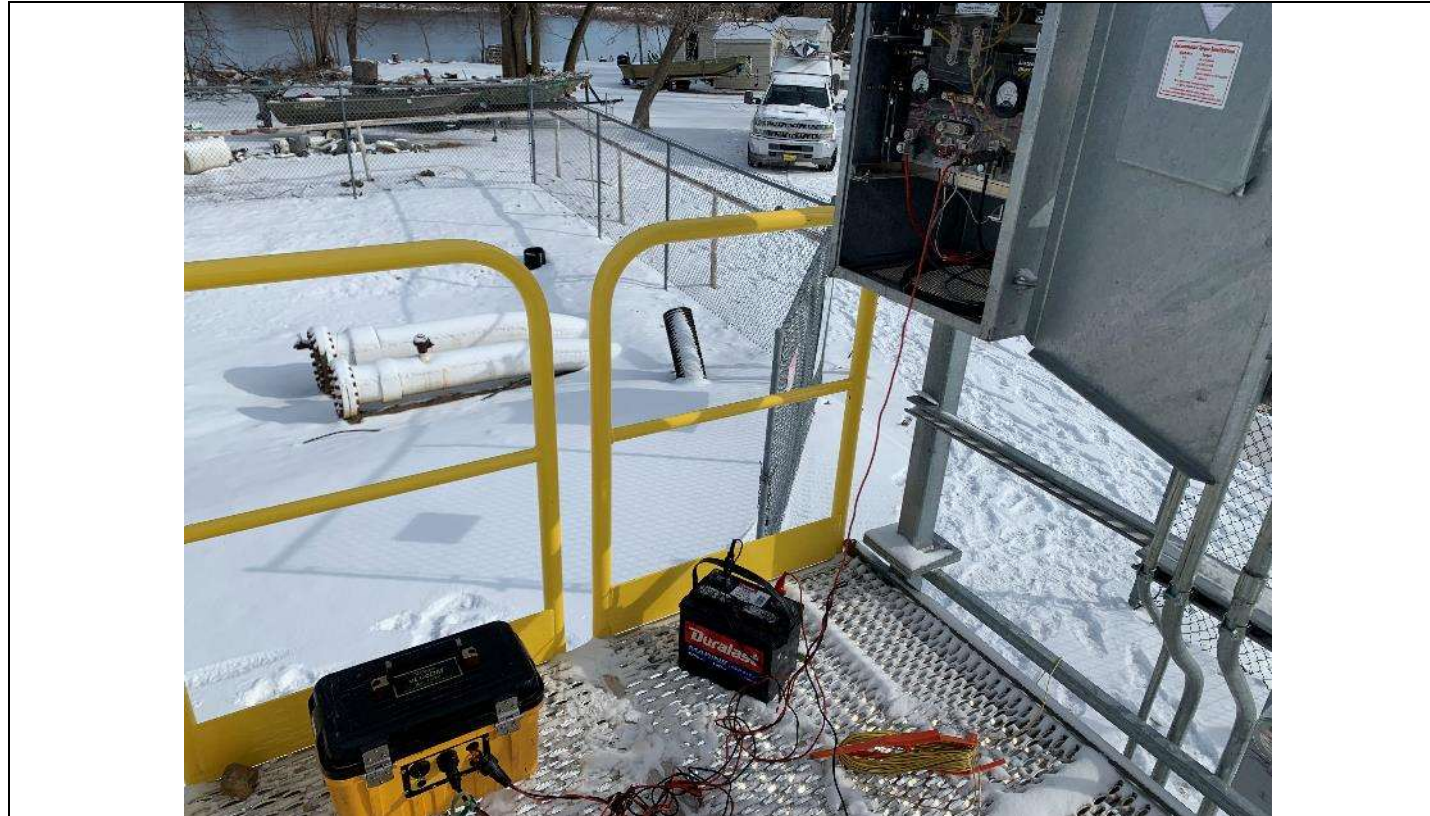
Transmitter Connection Site Overview
