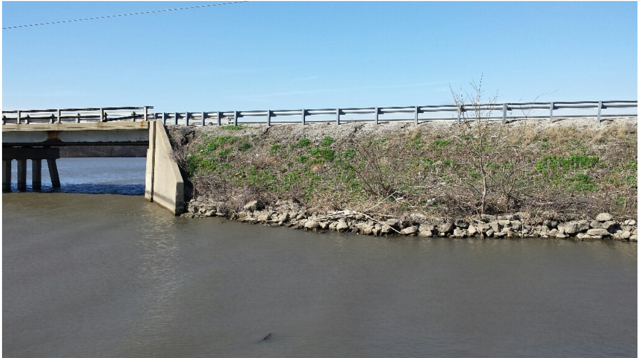
Photo 9 – Looking North At South Face of Roadway Embankment East of East Bridge
