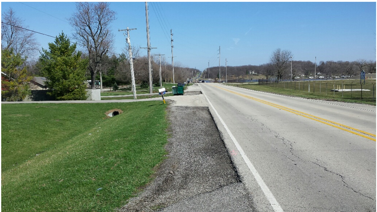
Photo 2 – Looking East Along North Side of Road from West End of Project
