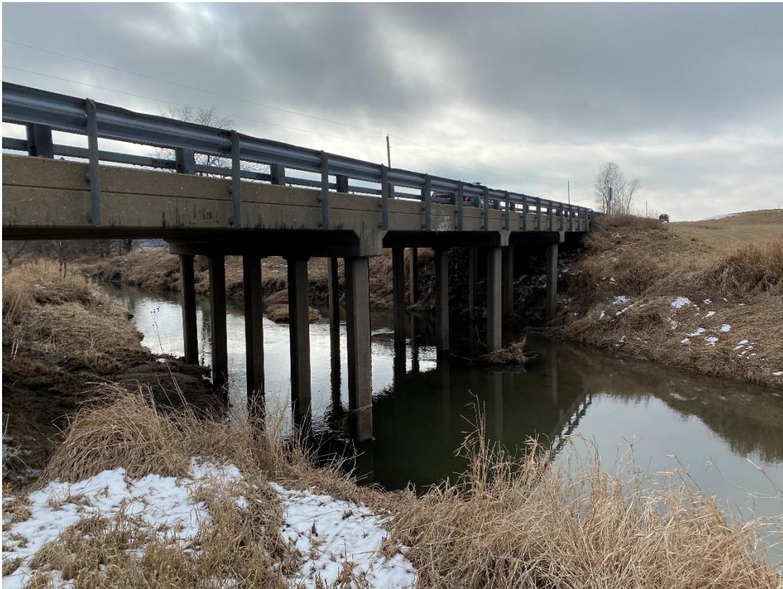
Photo 3. County Hwy 32/County Road 1000N (FAS 481) bridge, McLean County, Illinois, crossing Middle Fork Sugar Creek. Facing downstream at the north side of the bridge.
