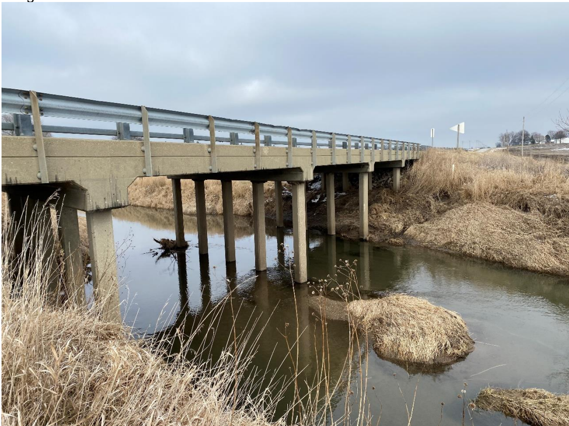
Photo 4. County Highway 32/County Road 1000N (FAS 481) bridge, McLean County, Illinois, crossing Middle Fork Sugar Creek. Facing upstream from south side of bridge.
