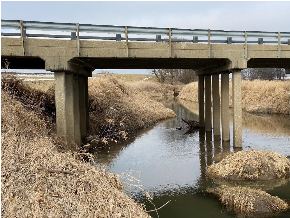
Photo 5. County Highway 32/County Road 1000N (FAS 481) bridge, McLean County, Illinois, crossing Middle Fork Sugar Creek. Facing upstream from south side of bridge.
