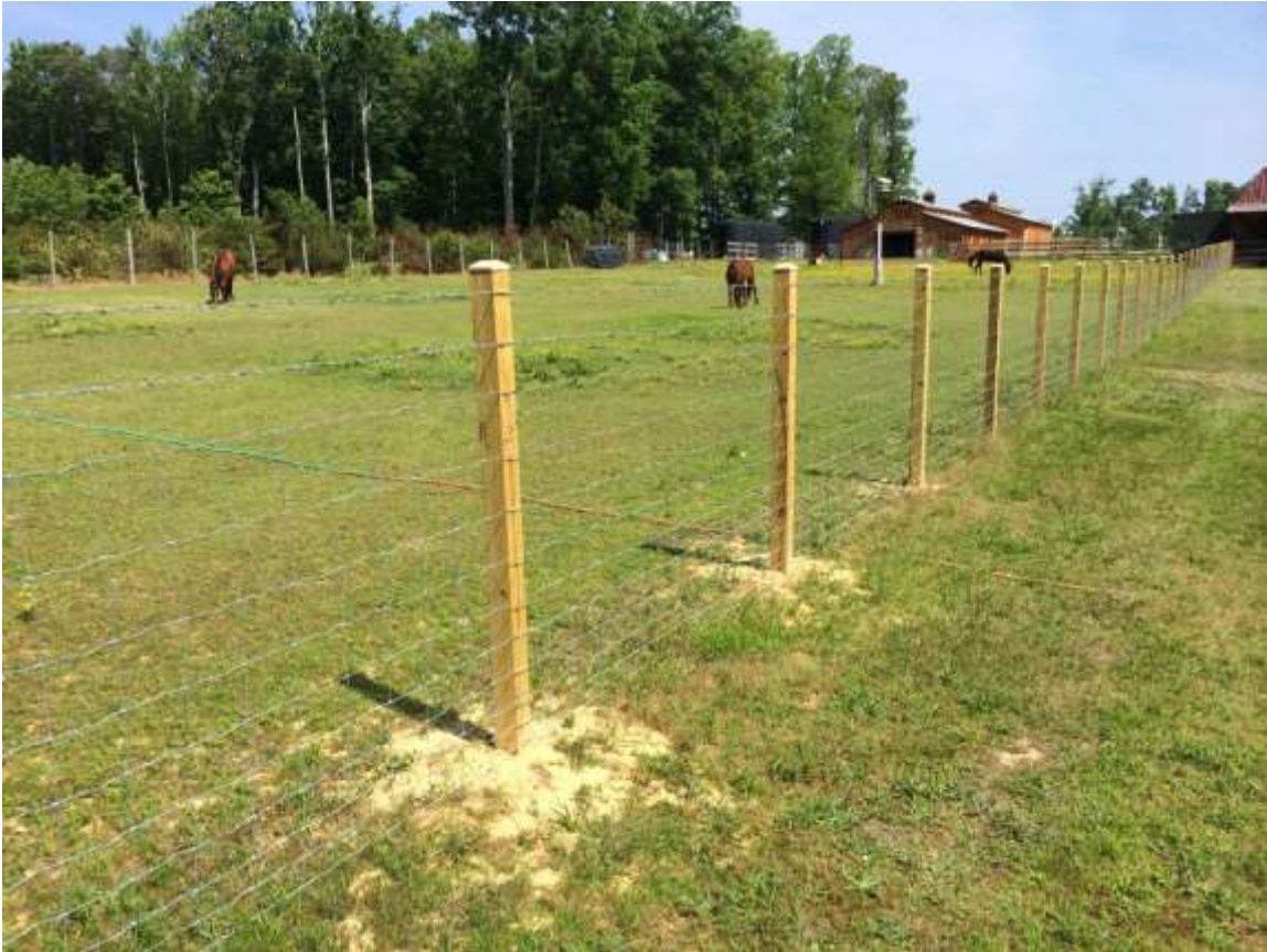
Example fence section. Planned fencing will be seven feet high and not include barbed wire.
