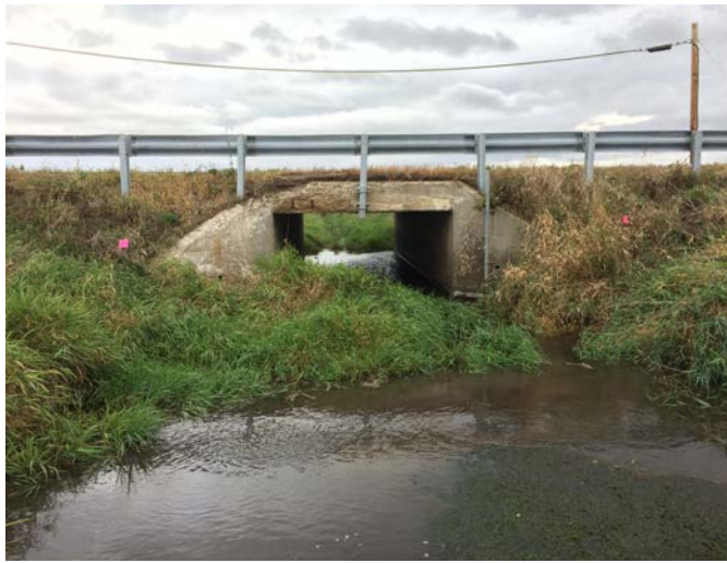
Photo 1: View of the west end of the Harmony Road over Harmony Creek culvert looking east.
