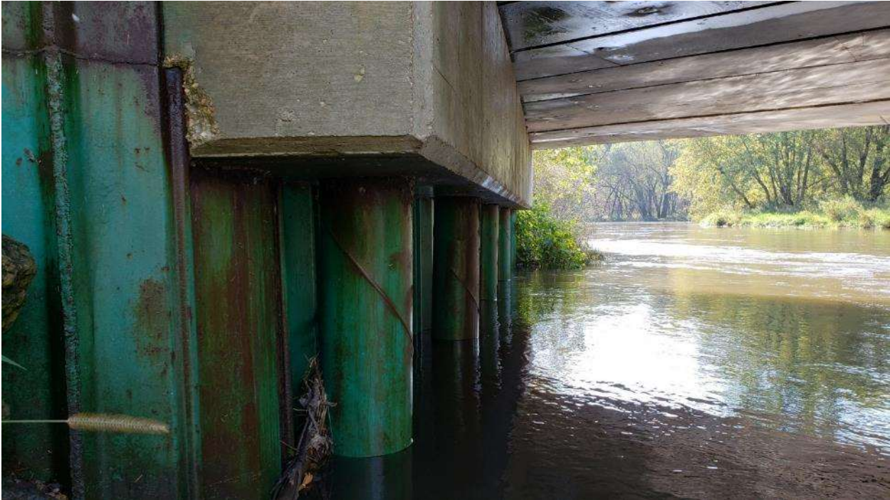
McNeal Rd at South Branch Kishwaukee River – Looking south at east abutment (Oct 2018).
