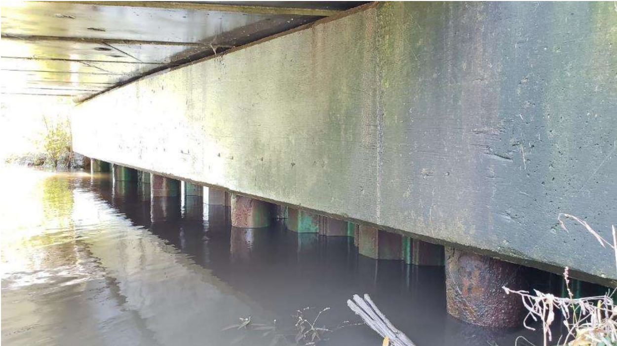
McNeal Rd at South Branch Kishwaukee R. – Looking southwest at west abutment (Oct 2018)
