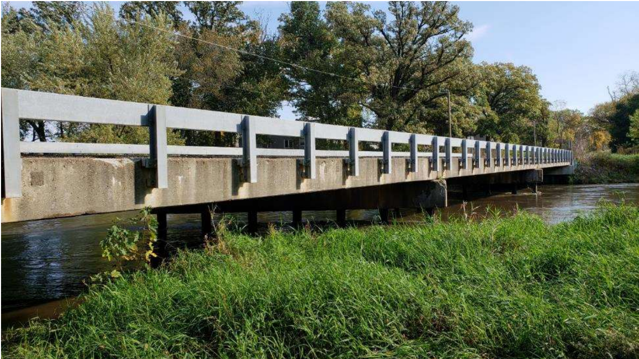
McNeal Road at South Branch Kishwaukee R. – South elevation looking northeast (Oct 2018).
