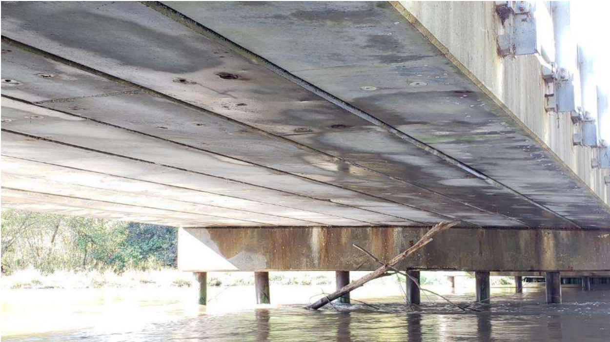
McNeal Rd at South Branch Kishwaukee River – Looking southwest at substructure (Oct 2018).
