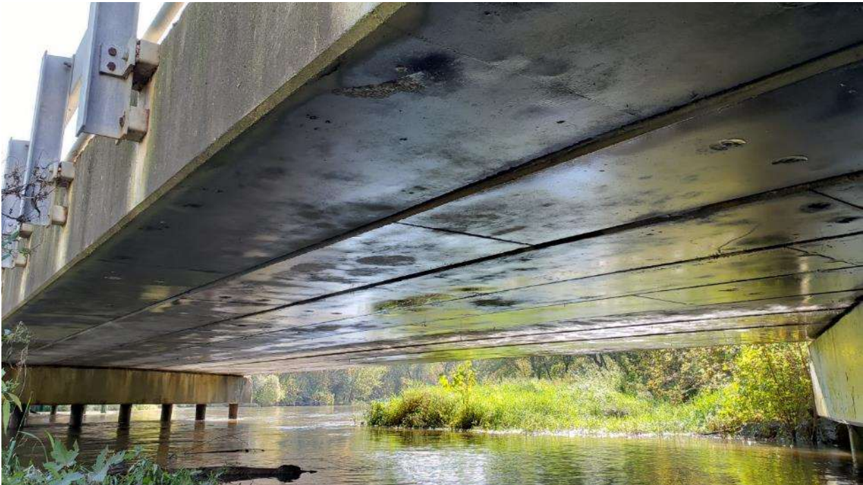
McNeal Road at South Branch Kishwaukee R. – Looking southeast at substructure (Oct 2018)
