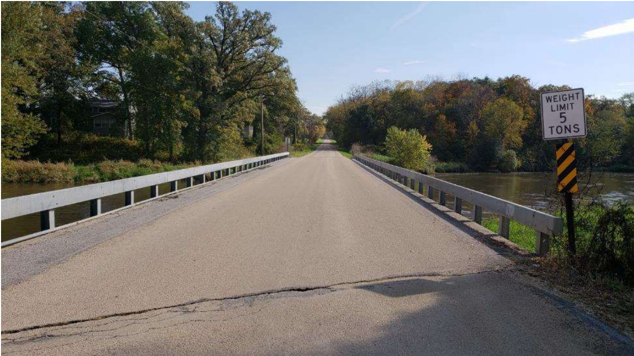
McNeal Road at South Branch Kishwaukee River – Looking east at bridge deck (October 2018).
