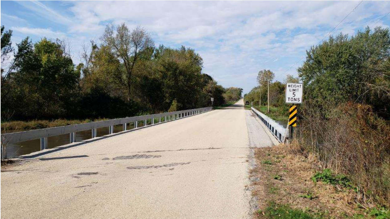
McNeal Road at South Branch Kishwaukee River – Looking west at bridge deck (October 2018)
