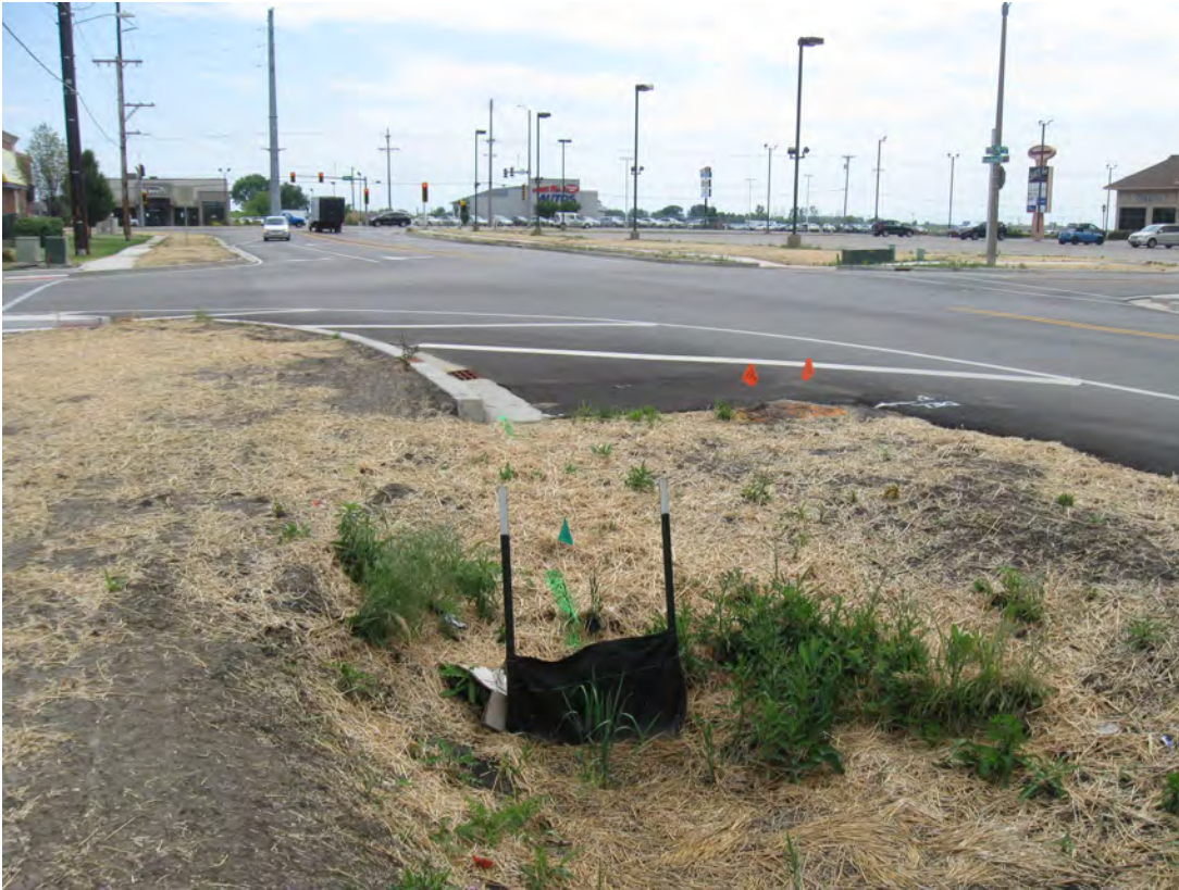
Intersection of Archer Elevator Road and HPR/Yucan Drive, looking south towards Wabash Avenue.
