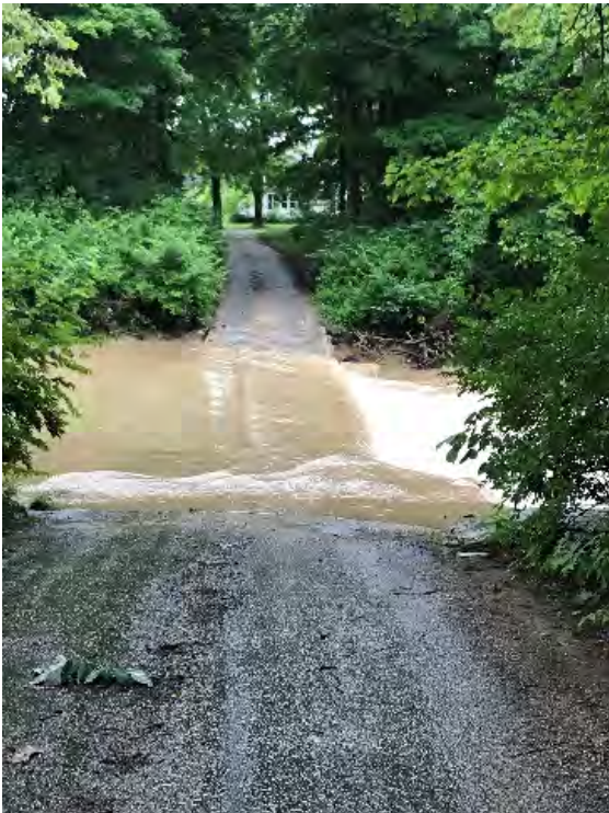
On Staley Road facing east; existing low water crossing (overflow culvert) under water.
