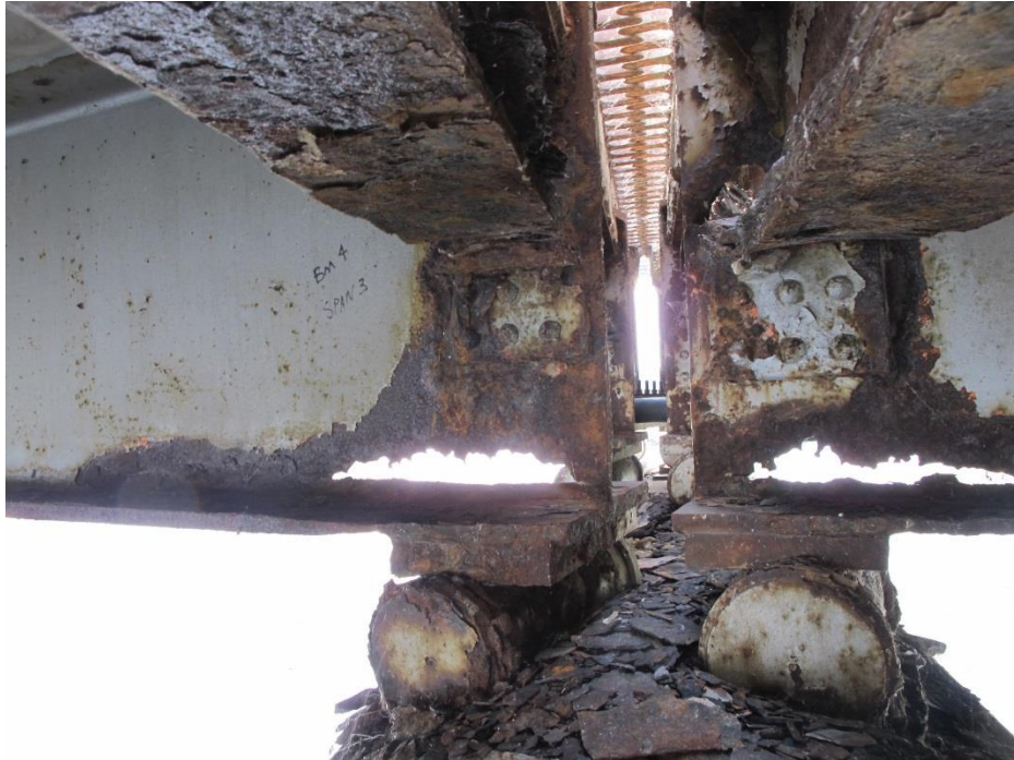
One example of severe corrosion in lower webs of beams and diaphragms (Pier 2, Beam 4 Shown)
