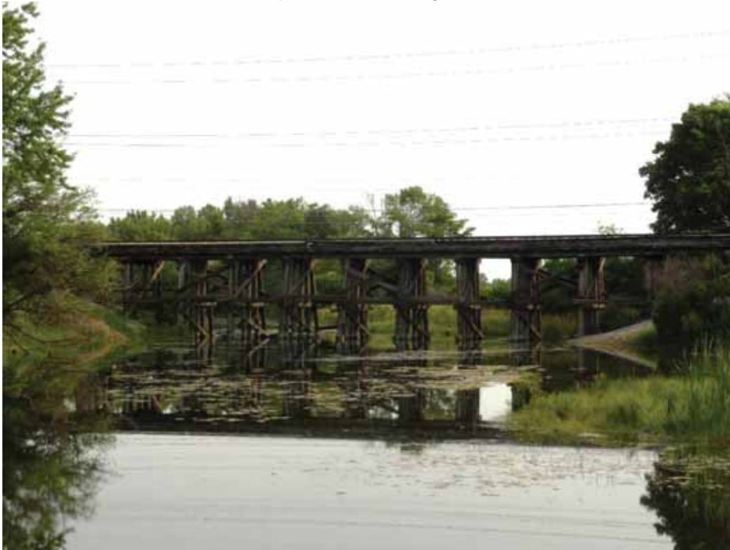
Plate 1. South side of the Freeport W 78.0 Bridge over the oxbow of the Kiswaukee River.
