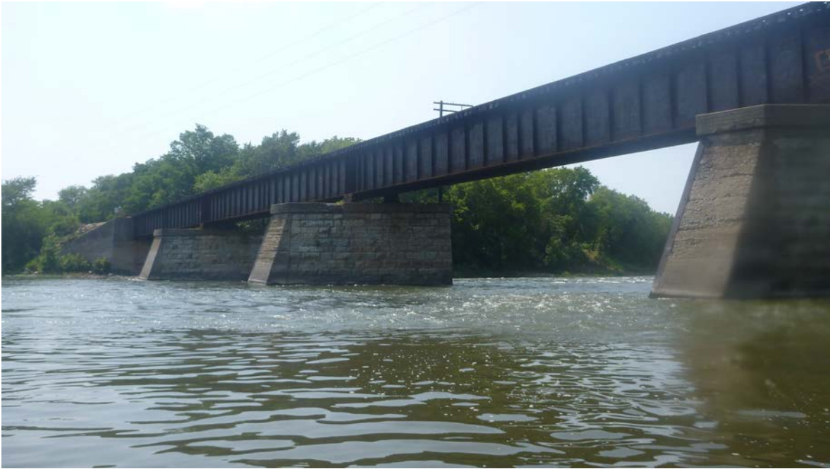
Figure 1. The National Railroad Passenger Corp. (AMTRAK) bridge over the Kankakee River (Wilmington, Will County, Illinois) where a freshwater mussel survey was conducted by INHS personnel on 21 July 2014. We sampled for mussels along the southeast shore above and under the bridge. (K.S. Cummings photo).
